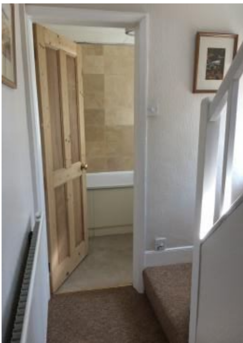
Bathroom at bottom of stairs with door width of 68cms
