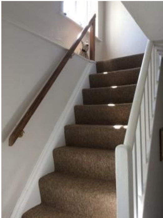
stairway with 2 handrails and window at the top giving good natural light. Width of the stairs is 81cms.
